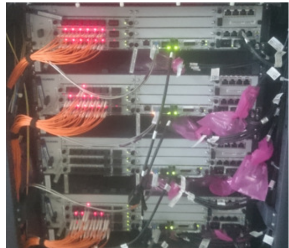
FIGURE 5: BBU pool used in TT central office location of C-RAN in Cekmekoy district of Istanbul.
