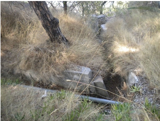
Fig. 14 Improper installation of the old surface drainage line
